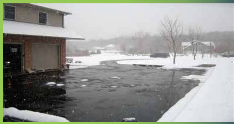
Snow Melt System After
